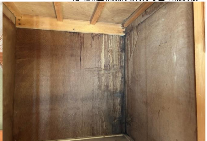
2階6帖和室(南側)押入壁の雨漏り痕
