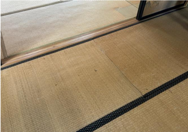
1階10帖和室床の沈み
